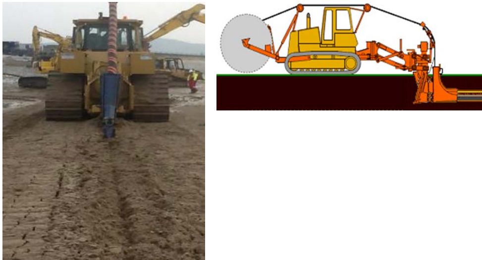
Figure 3 Above - Duct being installed by Plough method, Right – cross section of plough
